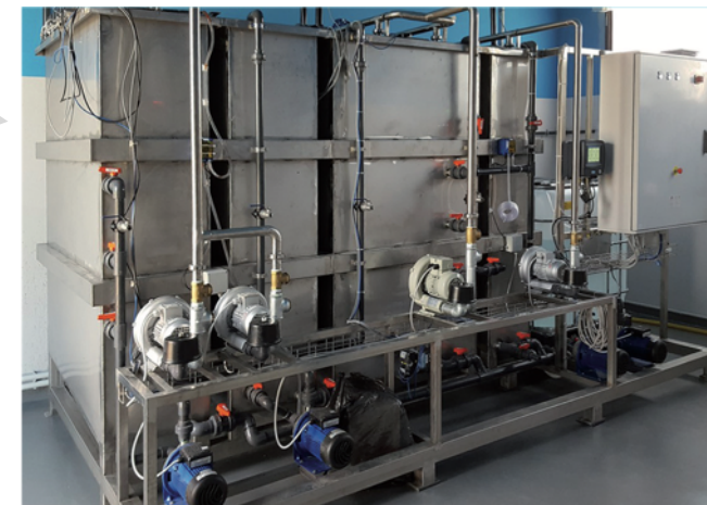
Pilot plant at the Carbonera WWTP (Italy)
